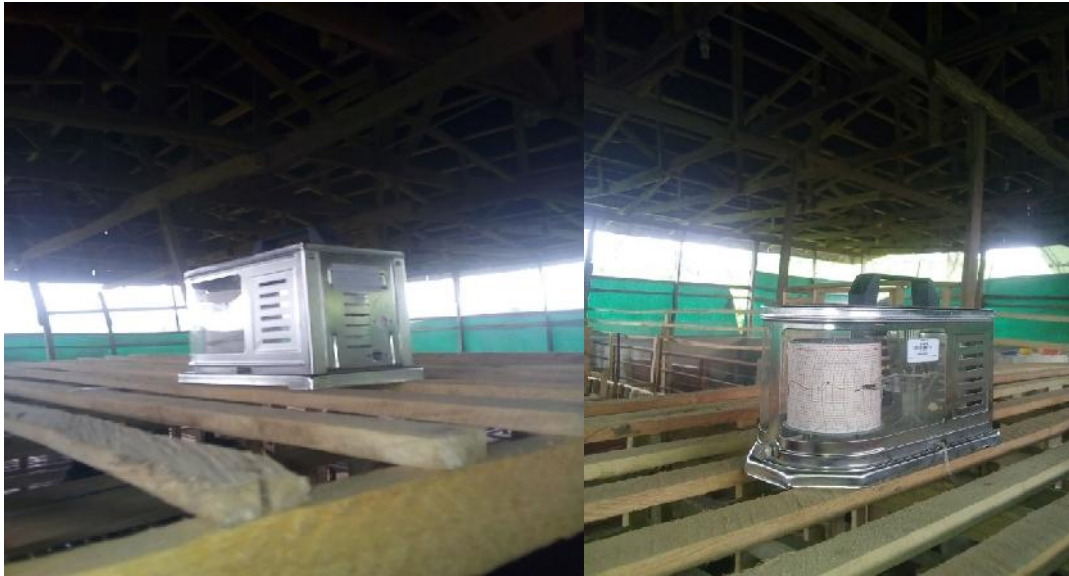
Figure 1: Automatic Temperature Humidity Measurement.
